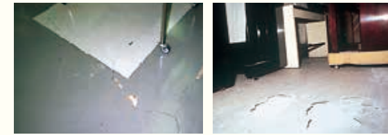
Cracks/peeling in laid flooring
